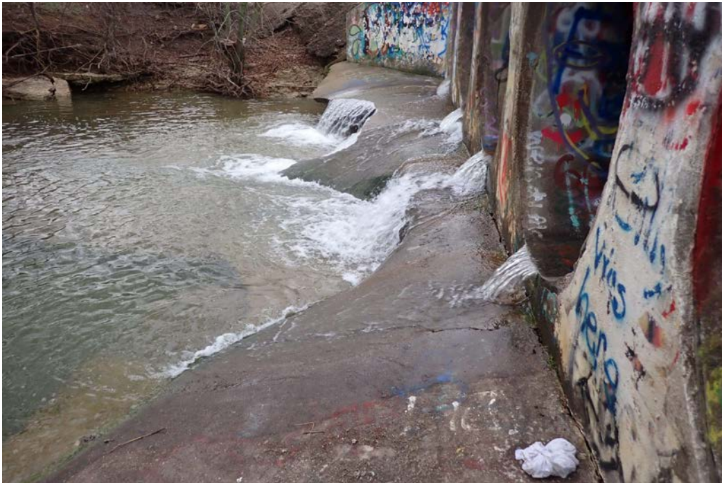
PHOTO 3 Condition Ratings of 4 or Lower, Recommended Maintenance Needs, Defect
