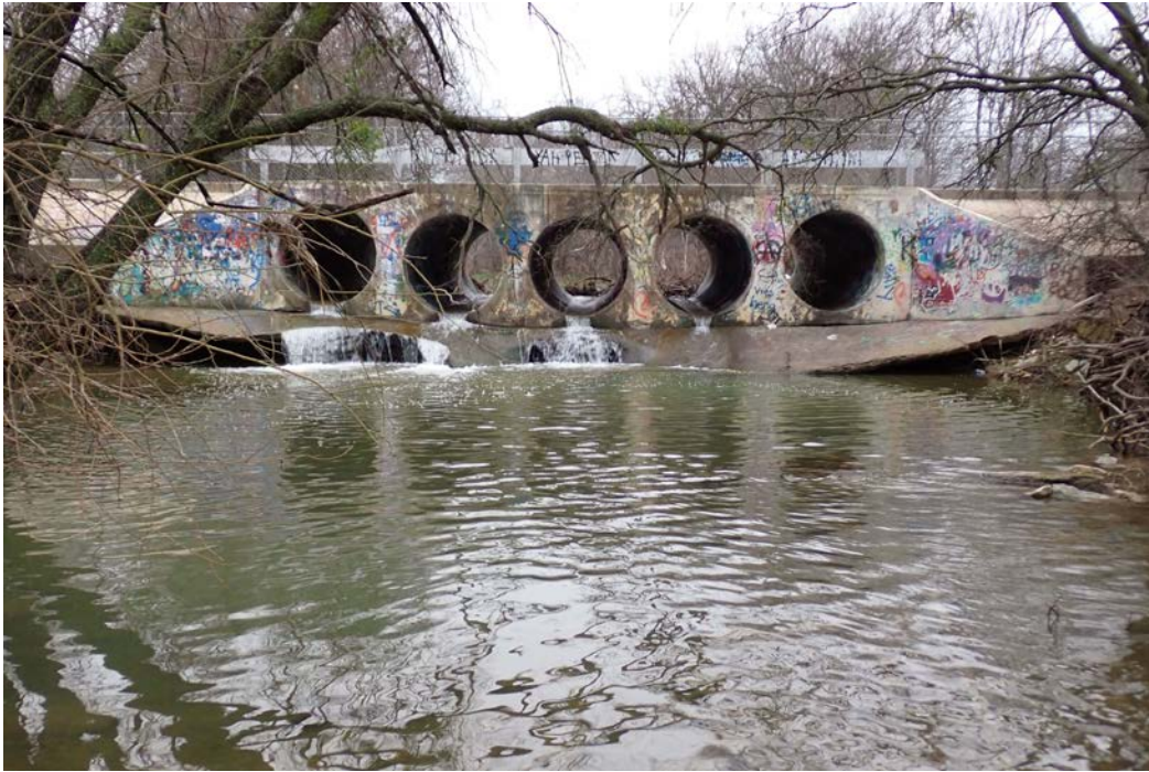
PHOTO 2 Stream Under View, Recommended Maintenance Needs, Defect
