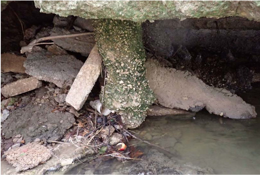
PHOTO 6 Condition Ratings of 4 or Lower, Recommended Maintenance Needs, Defect
