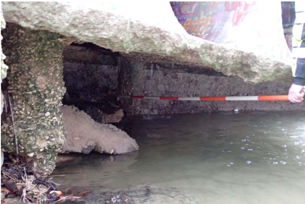
PHOTO 5 Condition Ratings of 4 or Lower, Recommended Maintenance Needs, Defect
