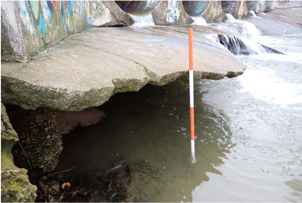
PHOTO 4 Condition Ratings of 4 or Lower, Recommended Maintenance Needs, Defect
