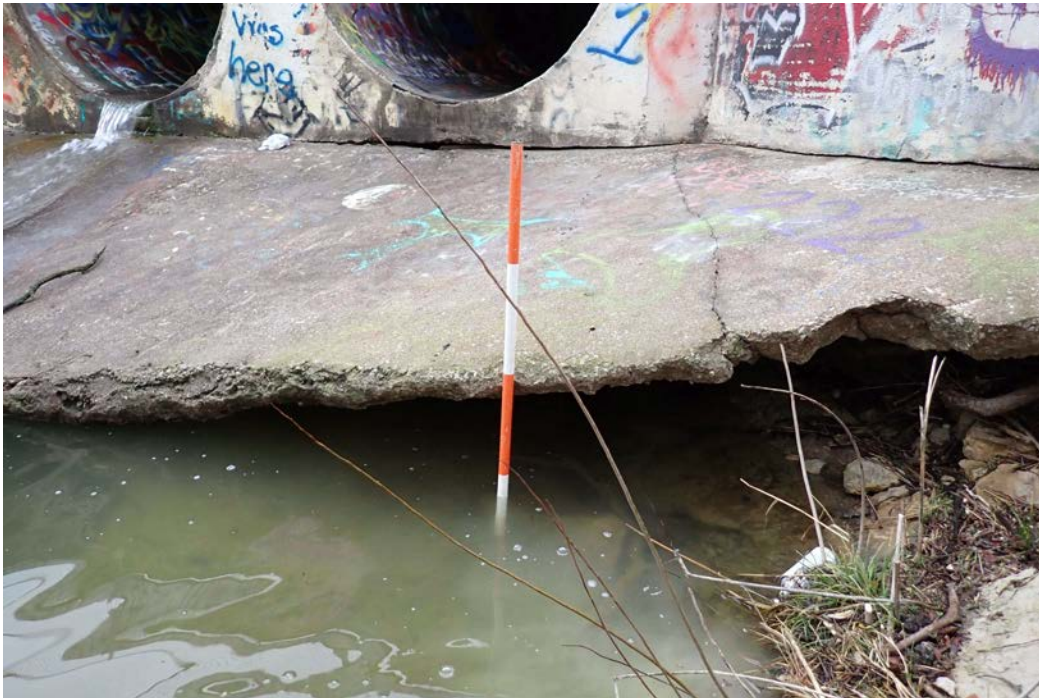
PHOTO 7 Condition Ratings of 4 or Lower, Recommended Maintenance Needs, Defect
